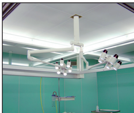
Theatre installation using Ref: 6 x 5SIF Multi
