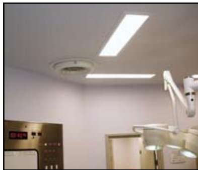
Operating Theatre luminaires supplied to Edgware General Hospital
