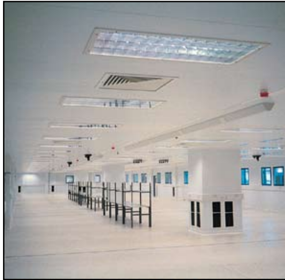
1200 x 600mm nominal recessed LG3/7 luminaires designed to fit a prepared aperture in a walk on foam ceiling system as supplied to this Oxford Electronics manufacturing Building
